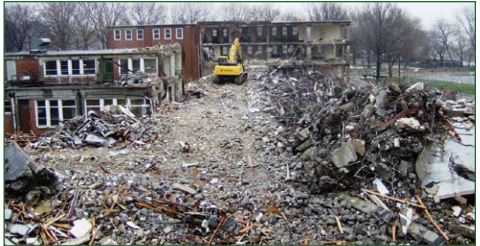
A crawler tractor from Charter Environmental Inc. works through debris from Building 408, a former barracks and law center at Fort Hamilton, N.Y. Photo courtesy of U.S. Army Engineering and Support Center, Huntsville, Ala.
